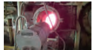
Facilities for processing insulating oil contaminated with low density PCBs (incinerated at over 1100°C)
