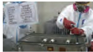
Workers extract oil at the storage facility for low density PCB contamination
