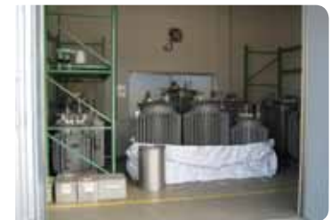
PCB storage rooms have all been moved to one room at the Head Office & Yokohama Business Center
