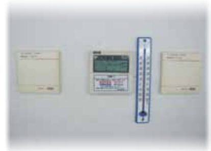
The temperature manager adjusts the AC while checking the room temperature
