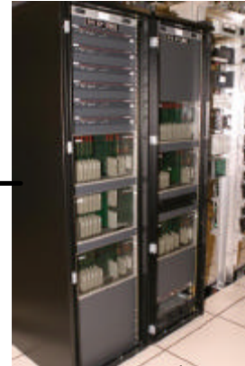
Zetron's Radio Controller
